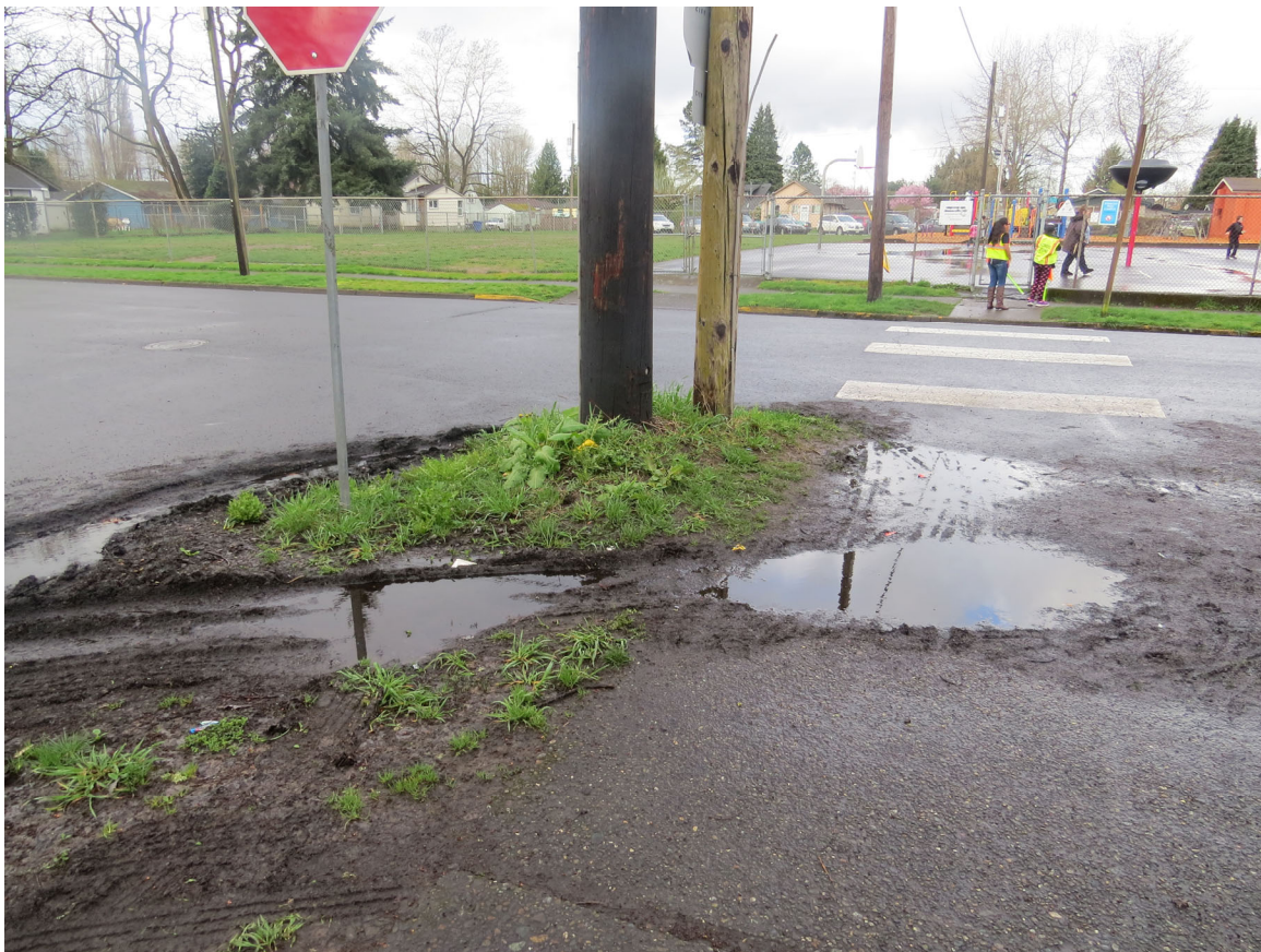
Missing sidewalk and corner ADA ramps
